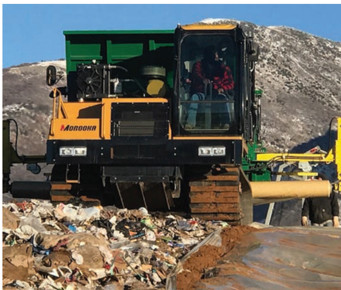
Davis Landfill's skilled operator lines up with film panels to create an overlap of the film for a complete barrier between the waste and environment.
