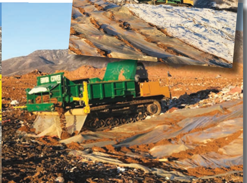
EPI's ECD 800 starting a new film panel run up a working face slope at Davis Landfill. The ECD 800 is capable of deploying film on 3 to 1 slopes.
